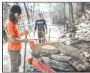
Back Solid Trail Construction workers Dean Russell (left) and Cason Vance pose rocks along a trail entry Thursday at Lake Matoka in Rogers. Rogers awarded a grant to update the trail around Lake Matoka. Check out more on www.ark.com/2022/01/26/back-solid-trail-construction/
