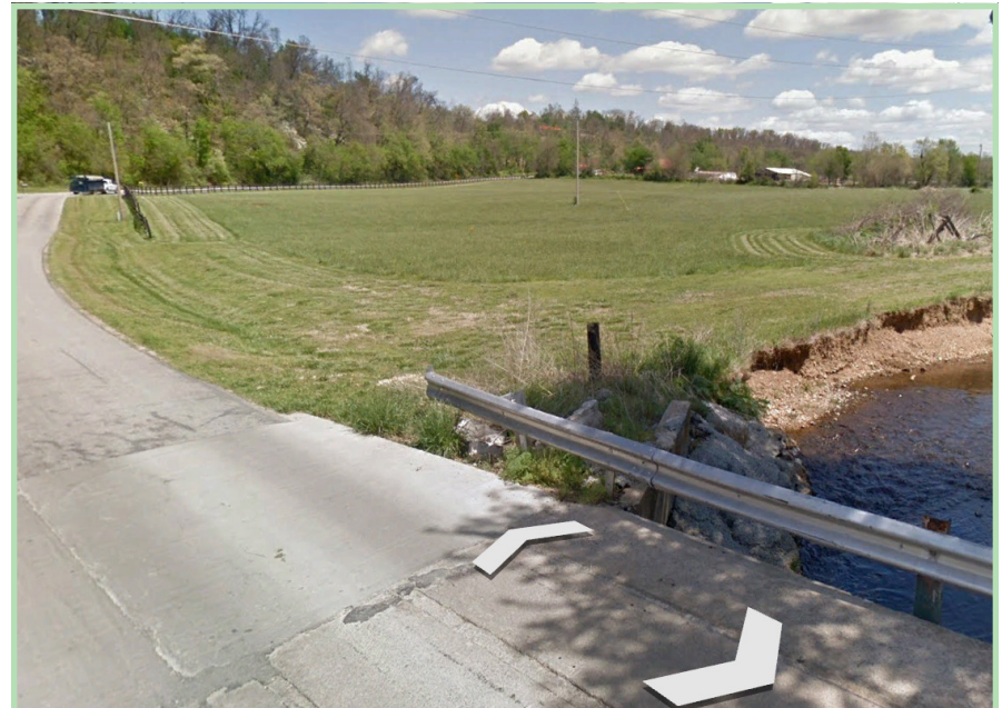
Brush Creek Rd at Brush Creek: An area of Rural near Rural Residential.
