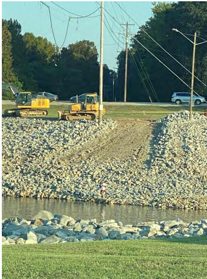
Figure 3-7. Repair in progress on Rankin County side (east) channel bank on October 6, 2023.
