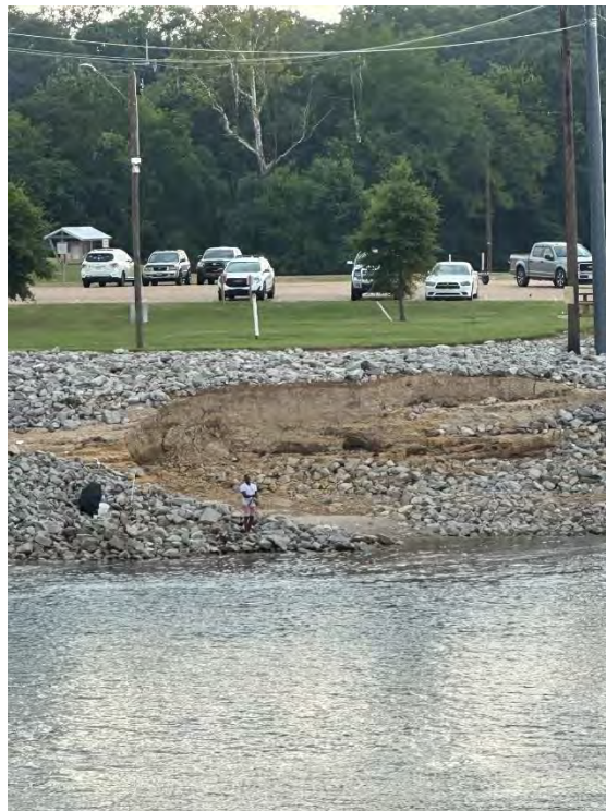
Figure 3-6. Scour on Madison County side (west) channel bank on July 10, 2023
