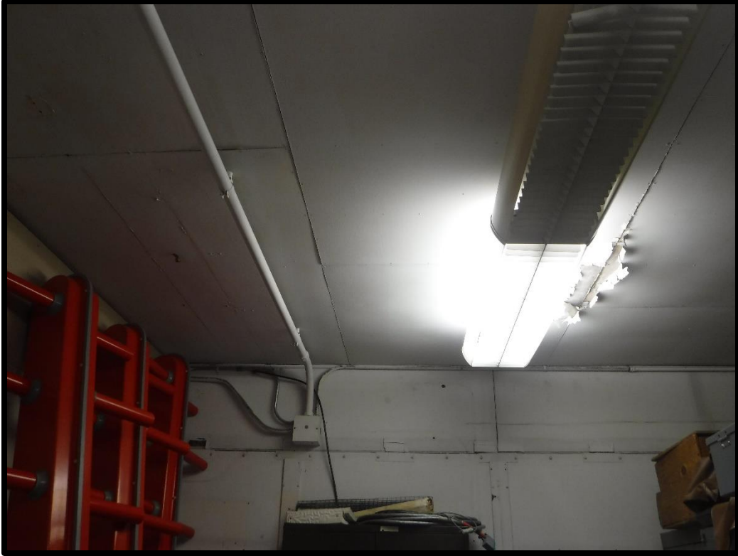
Figure 12. View of Equipment Room ceiling and wall of Little Rock VORTAC building
