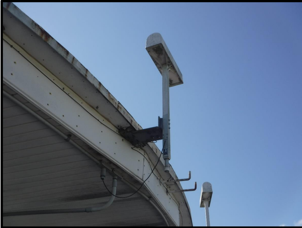
Figure 9. View of Monitor Antenna on Western façade of Little Rock VORTAC building (facing south-southeast)
