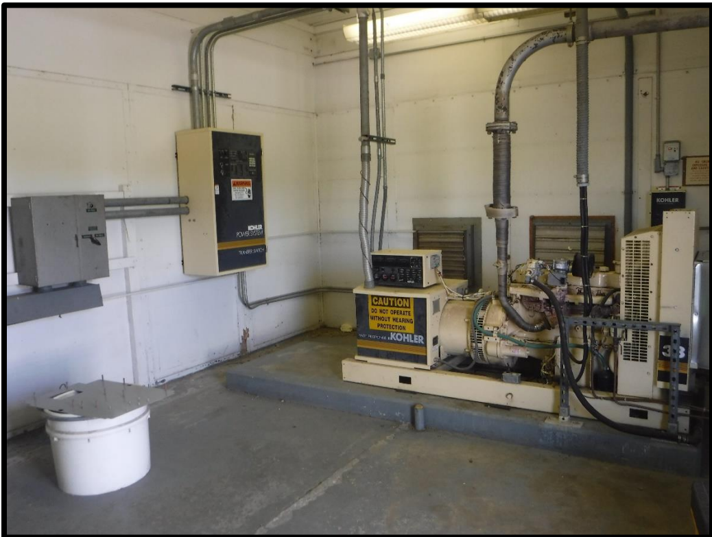
Figure 13. View of Generator Room of Little Rock VORTAC building
