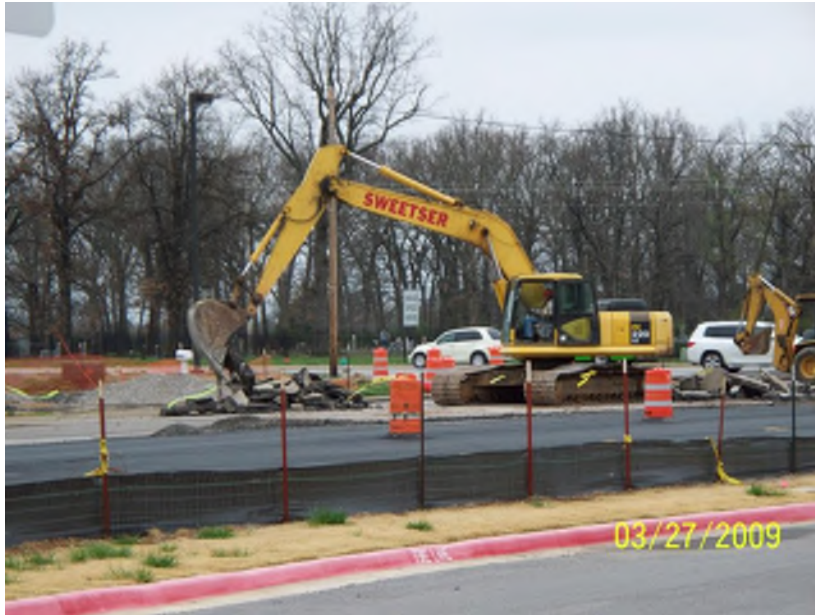
Photograph CS-4 – Example of Silt Fencing
