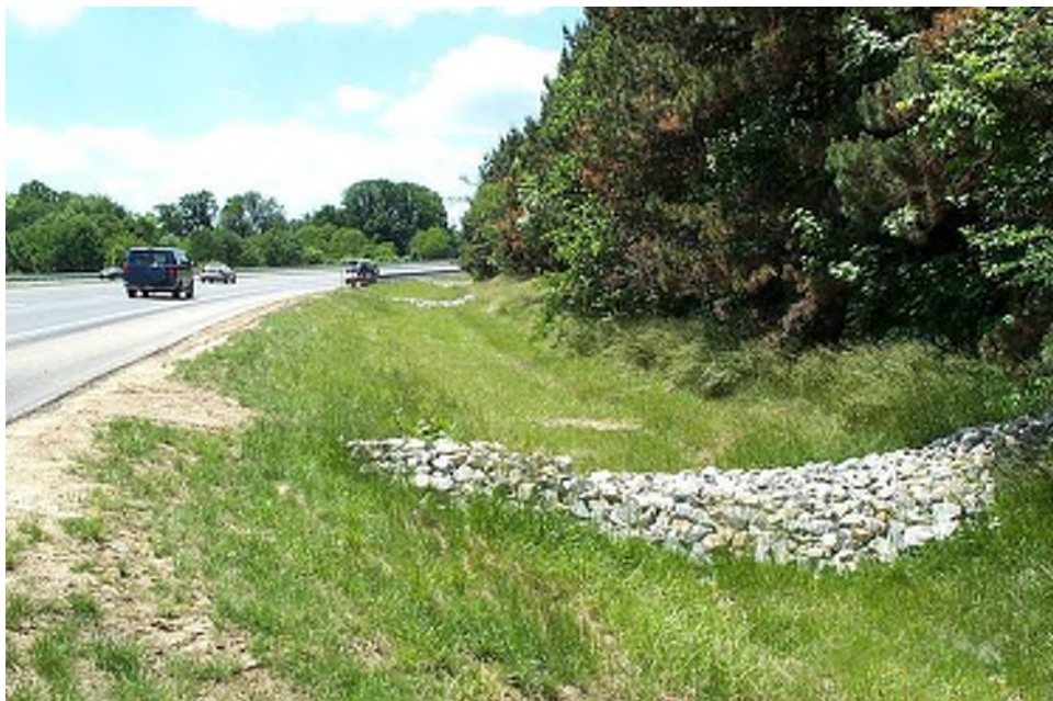
Photograph CS-8 – Example of Rock Check Dam (Source: Delaware DOT)
