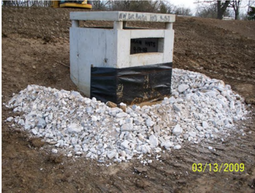
Photograph CS-5 – Example of Inlet Protection
