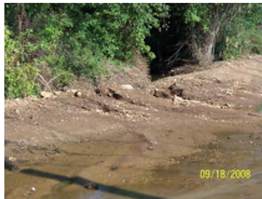
Photograph CS-1 – Example of Erosion during Construction
