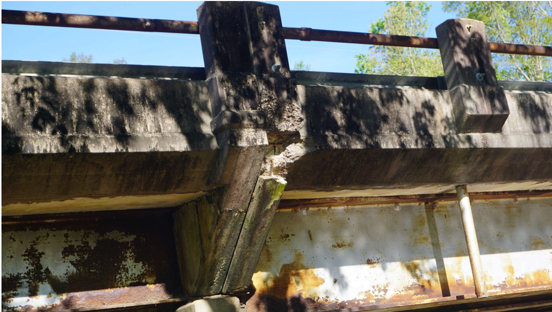
PHOTO 9 Deck Description BRIDGE RAIL SPALLED.
