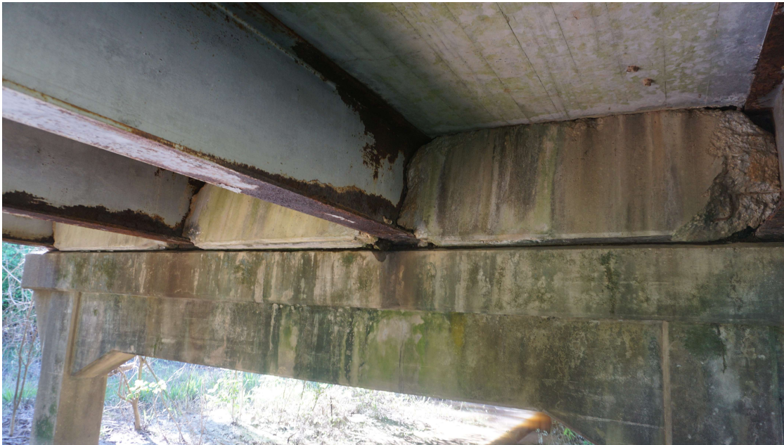
PHOTO 6 Superstructure Description DIAPHRAGMS SPALLED ABOVE CAP.
