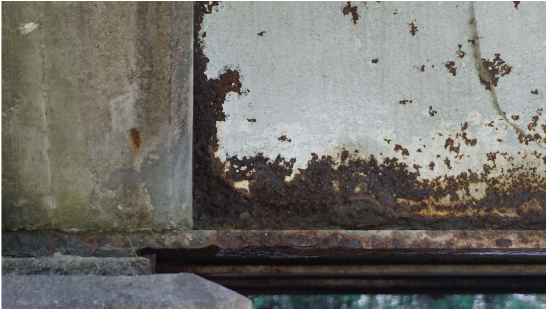
PHOTO 5 Superstructure Description BEAM ENDS SEVER RUSTING.
