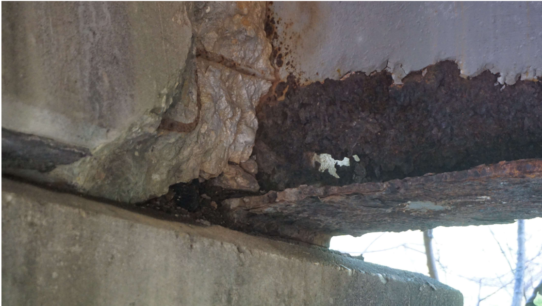
PHOTO 7 Superstructure Description SECTION LOSS IN BEAM, WITH DIAPHRAM SPALLED.
