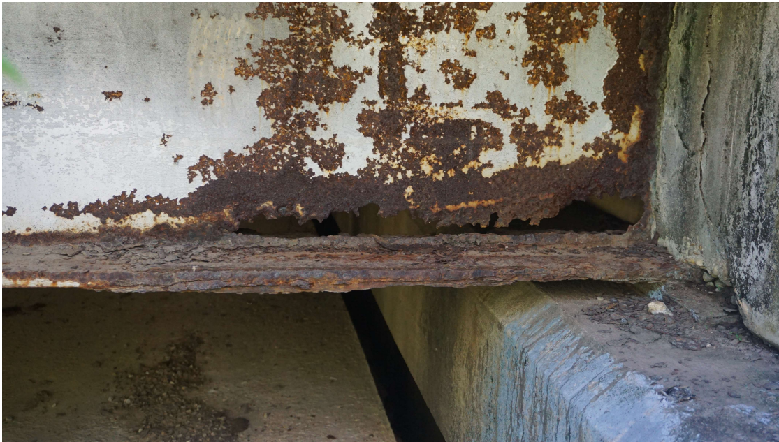
PHOTO 4 Superstructure Description HIGH SECTION LOSS IN BEAM.
