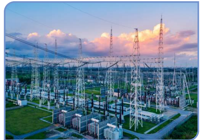
high voltage substation
