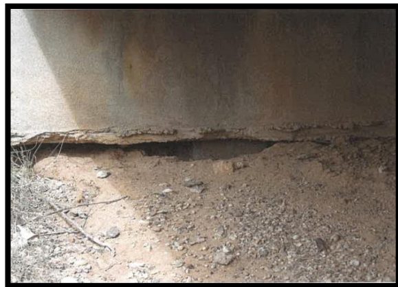
Figure 10: 17589 Scour of the base
