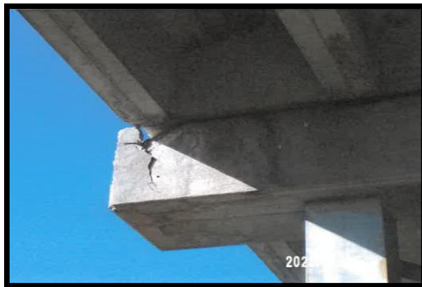
Figure 9: 17589 Spalling in cap, exposed rebar
