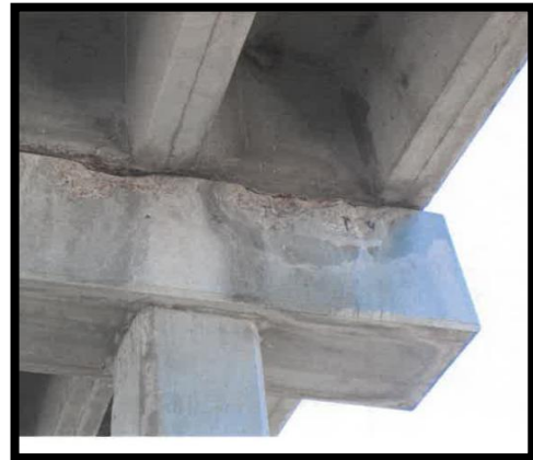
Figure 6: 15210 Spall in cap and exposed rebar
