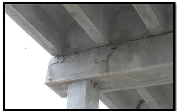
Figure 8: 17606 Spalling in cap and signs of delamination
