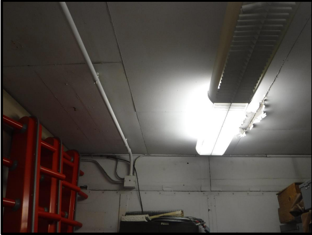
Figure 12. View of Equipment Room ceiling and wall of Little Rock VORTAC building
