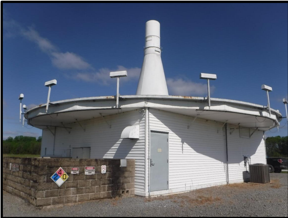
Figure 5. View of Southern and Eastern façades of Little Rock VORTAC building (facing northwest)
