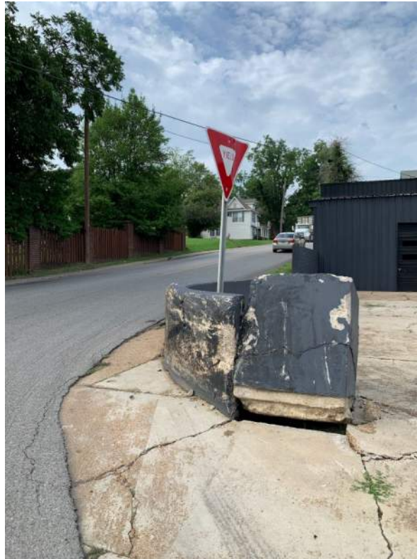
Figure 6: Damaged retaining wall in 90-degree bend intersection of Hwy 90
