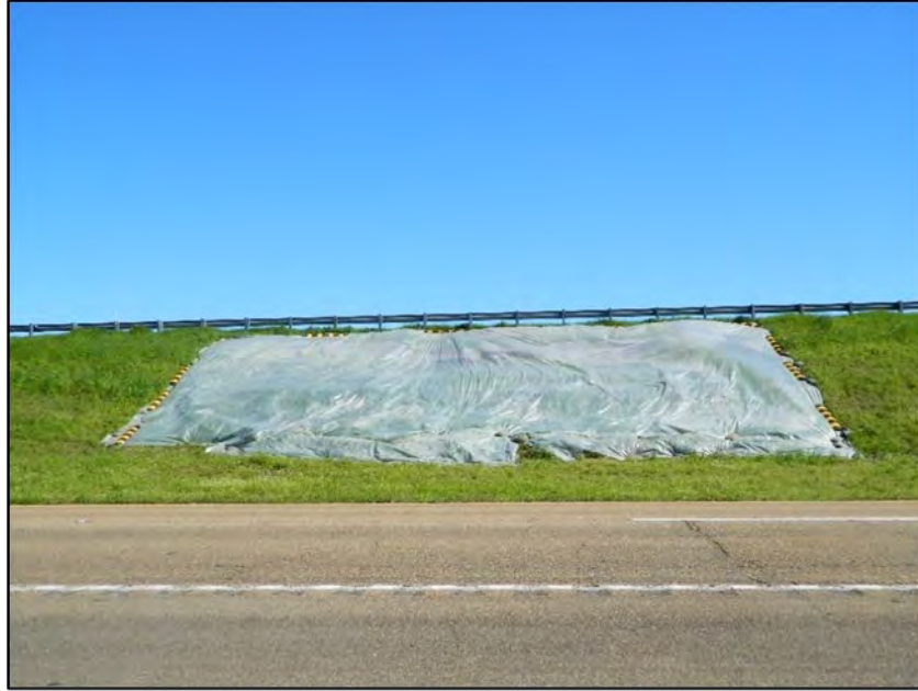
Figure 6 - Maintenance of a slide on the east side of the Dam (March, 2020).
